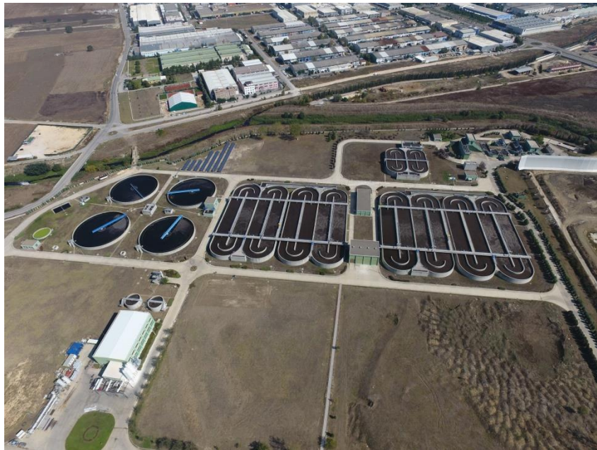
Example of Sewage Disposal (Bursa Uludag University, Turkey) : Wastewater treatment plant of the city that receives the sewage generated by Bursa Uludag University
